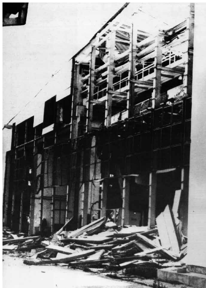
150. Al Soko in Mostar, Composite technologies hall, southern industrial zone (the right bank of the Neretva)
