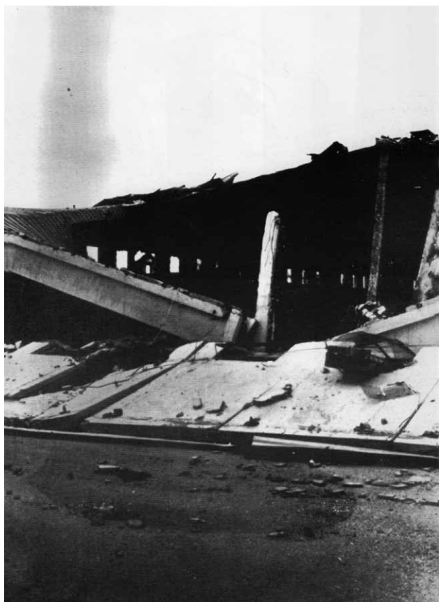
153. Cigarette Factory in Mostar, the destroyed warehouse, southern industrial zone (the right bank of the Neretva)
