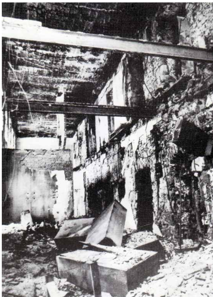
107. Vakufski Court (today PE "Prostor"), interior, the middle city belt (the left bank of the Neretva, Braće Fejića Street), year 1894
